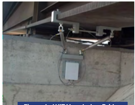
Figure 6a LVIT Mounted on Bridge
